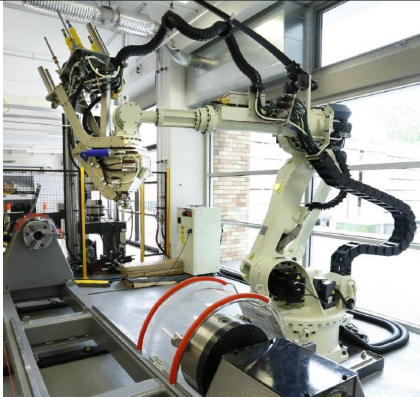
Figure 2.1 AMAC's Automated Fibre Placement facility located at UNSW
